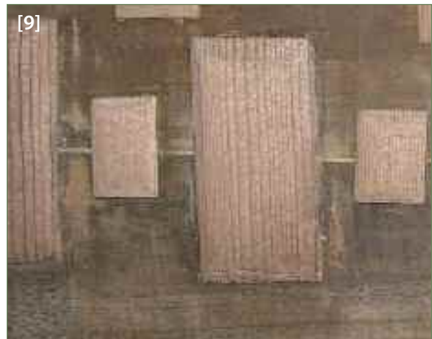
[9] The repaired crack reinforced with cleats
