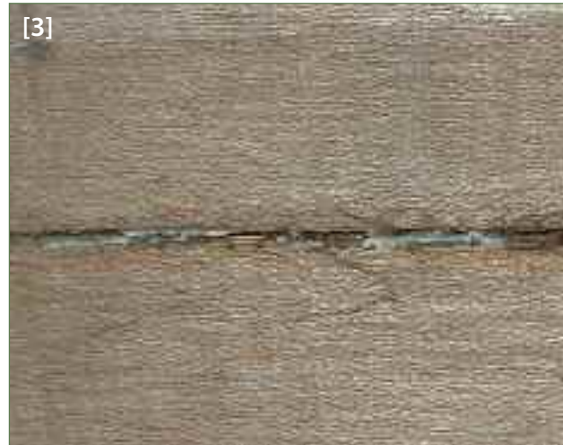
[3] Old synthetic glue can be seen in the crack prior to its repair
